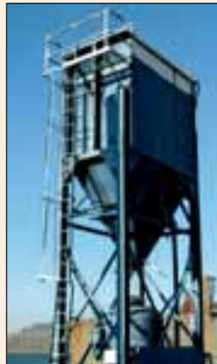
View of Sandblast Hopper & Tank
