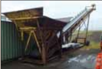
Load Out Conveyor Located at Vancouver, Washington Facility
